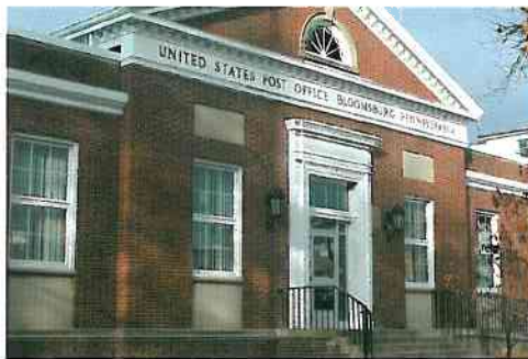
Bloomsburg USPS, Bloomsburg, PA The project consists of removing exterior wood trims from the entire building and replacing the trim with “Fypon” material.
